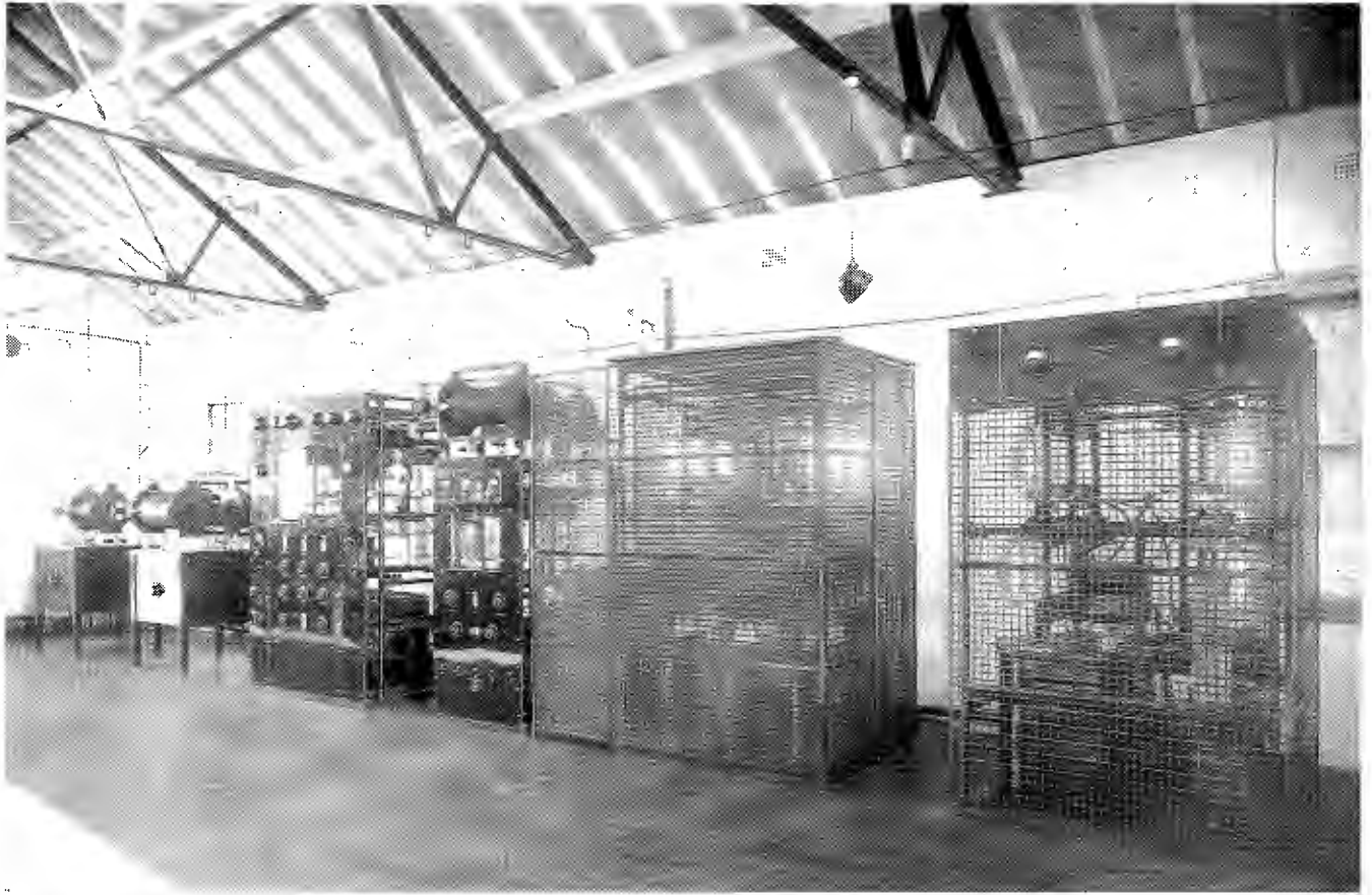
The original 5-kilowatt transmitter used by 2FC, pictured in the Pennant Hills transmitter hall. It was designed and built by AWA engineers Joseph Griffiths Reed and George Cookson, under the direction of chief engineer Arthur Stephen McDonald.
